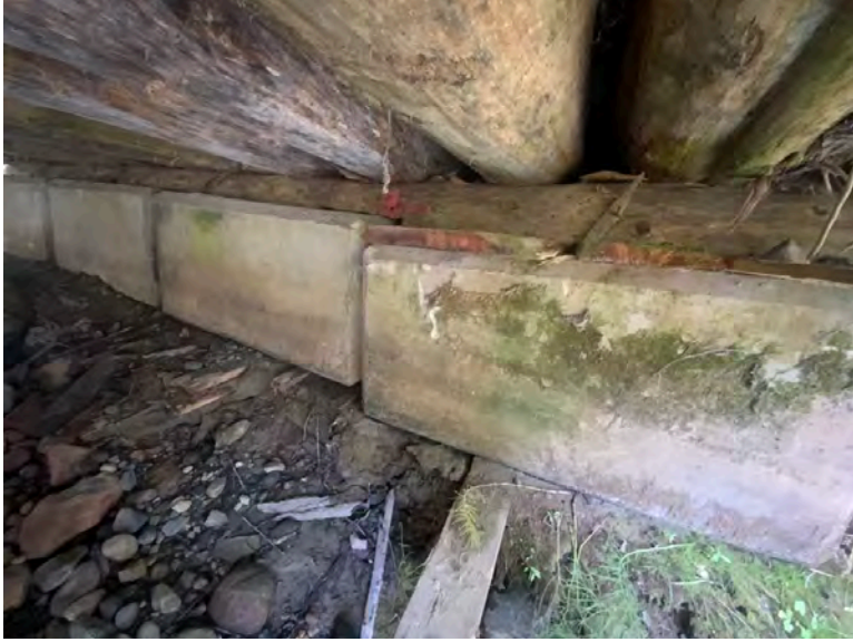
Shimmed locblock woods side due to block settlement
